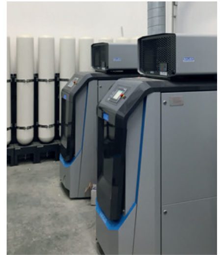
VERTICUS systems in operation at cooling specialist Guntner
